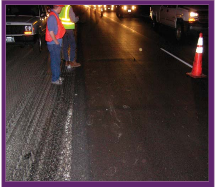
Inspection of the Warm Mix Asphalt (WMA) as it is placed on a CDOT project on Interstate 70.
